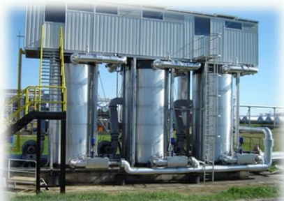
INA , 3 x VKS 5000 Thermal oil heater 3 x 5 MW
