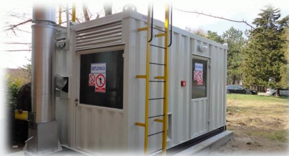
VUPIK d.d., Vukovar, Steam container boiler room, VPS 300 - 300 kg/hr - 2,7 bar
